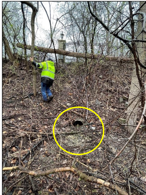
Photo 10 – Outlet pipe from control structure east of driveway for 381 County Line Road
