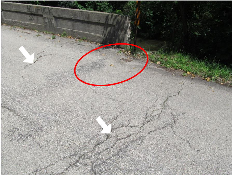
Figure 5. Settlement of approach pavement at the southeast corner of the bridge deck (arrow) and transverse cracking of the asphalt pavement (arrows).
