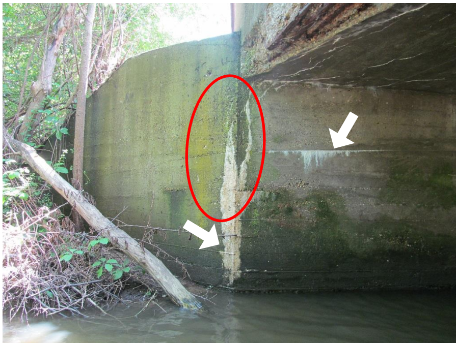
Figure 8. South abutment showing areas of efflorescence (arrows) and delamination (circle).
