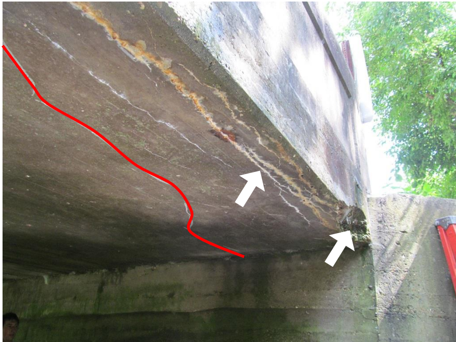
Figure 4. Spalled concrete and efflorescence (arrows) at southwest corner of the deck soffit (red line shows extent of delaminated concrete).
