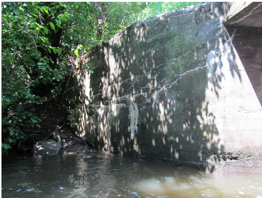
Figure 6. Freeze/thaw damage on the northwest wingwall, including cracking with efflorescence.
